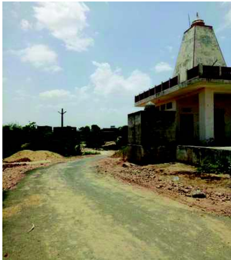
Figure No.-5.2(A) Newly constructed access road for getting access to the temple
