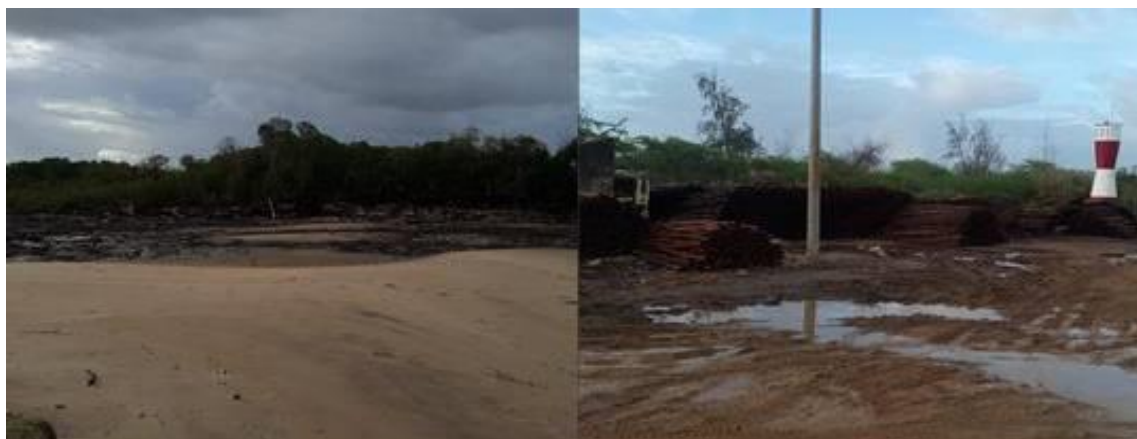
Plate 22: On-Going Mangrove Forest Clearance to Create Space for LAPSSET Corridor in Lamu
