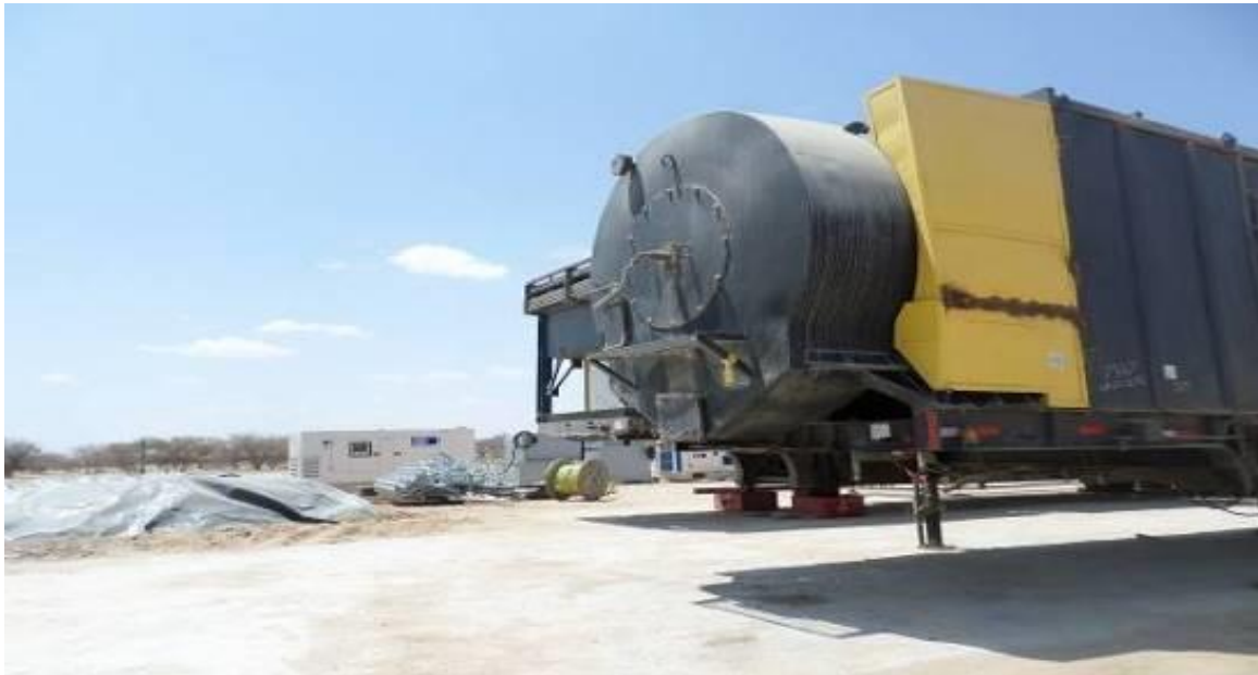
Plate 26: Thermal Desorption Unit in Machakos County (near Nairobi)
