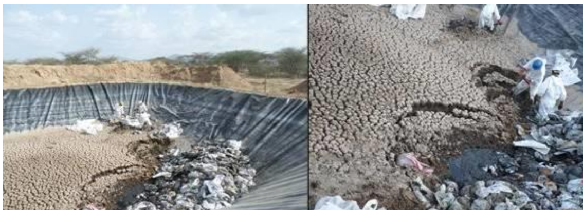
Plate 24: Existing Temporary Storage Facilities for Hazardous Oil Drill Waste in Turkana
