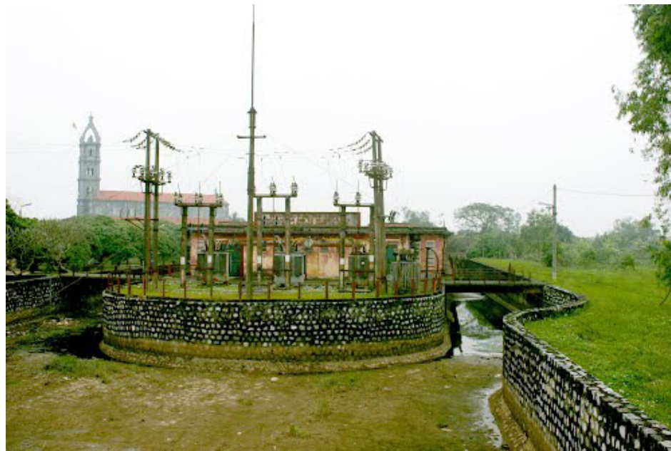
Figure 2-3. Chanh River Drainage Pumping Station
