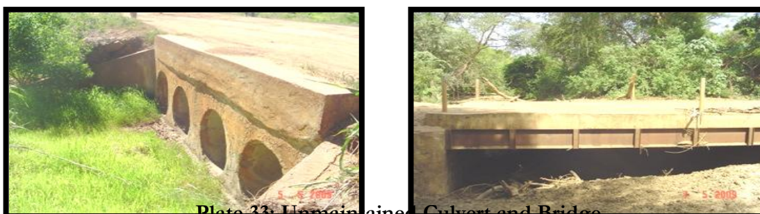
Plate 33: Unmaintained Culvert and Bridge
