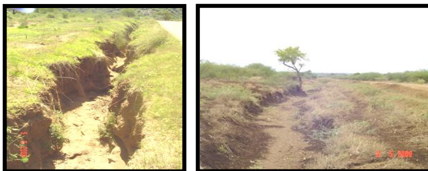
Plate 35: Erosion Gullies along the Road
