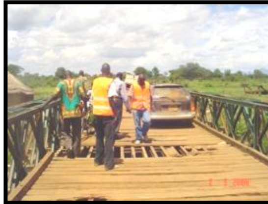
Plate 42: A Section of Dilapidated Bridge
