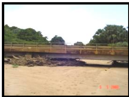
Plate 34: Kidepo Bridge Blocked by Sand and Debris
