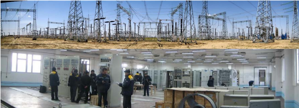
Figure 2.2. Completed Talimarjan Switch Station
