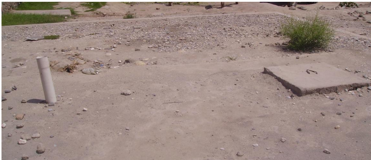
Wastewater tanks built for liquid waste on the site of the new lab in Jalalabad.
