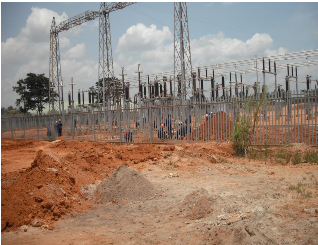
Plate 2.7: Sub Station works under construction at Kawanda and are likely to be similar to that at Kinyara and Hoima (Bulemwa village)
