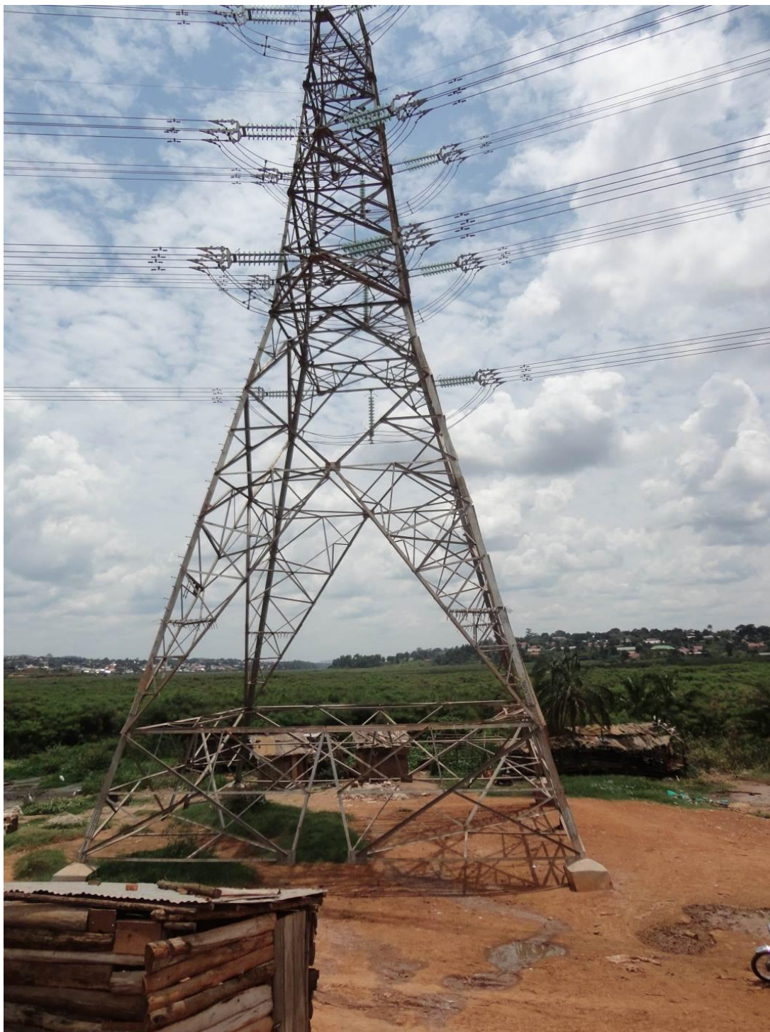
Plate 2.6 A fully operational 220kV lattice tower
