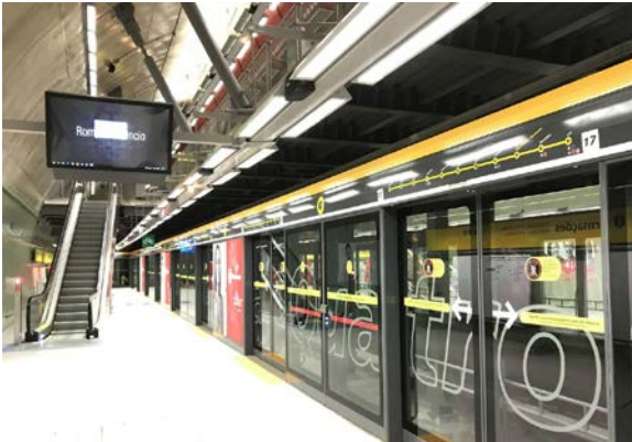
Platform doors in Higienopolis-Mackenzie station
