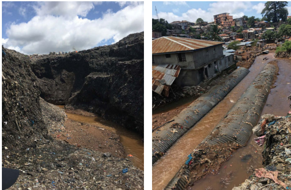
PHOTO 3: Granville Brook Running through Dump Site and Culvert Immediately Downstream of Dump Site
