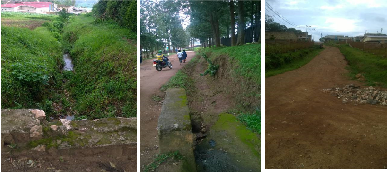
Plate 6: D1 above as an existing drainage along R15 and R 16 road at Kavumo Village, Gitarama Cell
