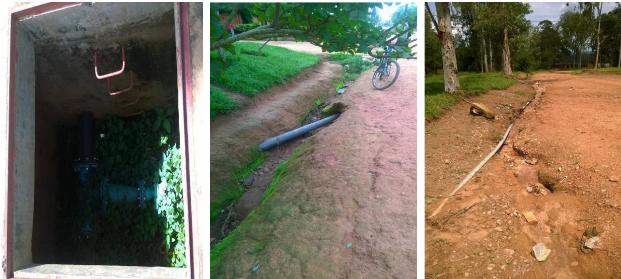
Plate 5: Drainage systems D1, D4, D5 and D6 need to be rehabilitated as their current state has resulted into storm water eating into the roads R2 and R1.
