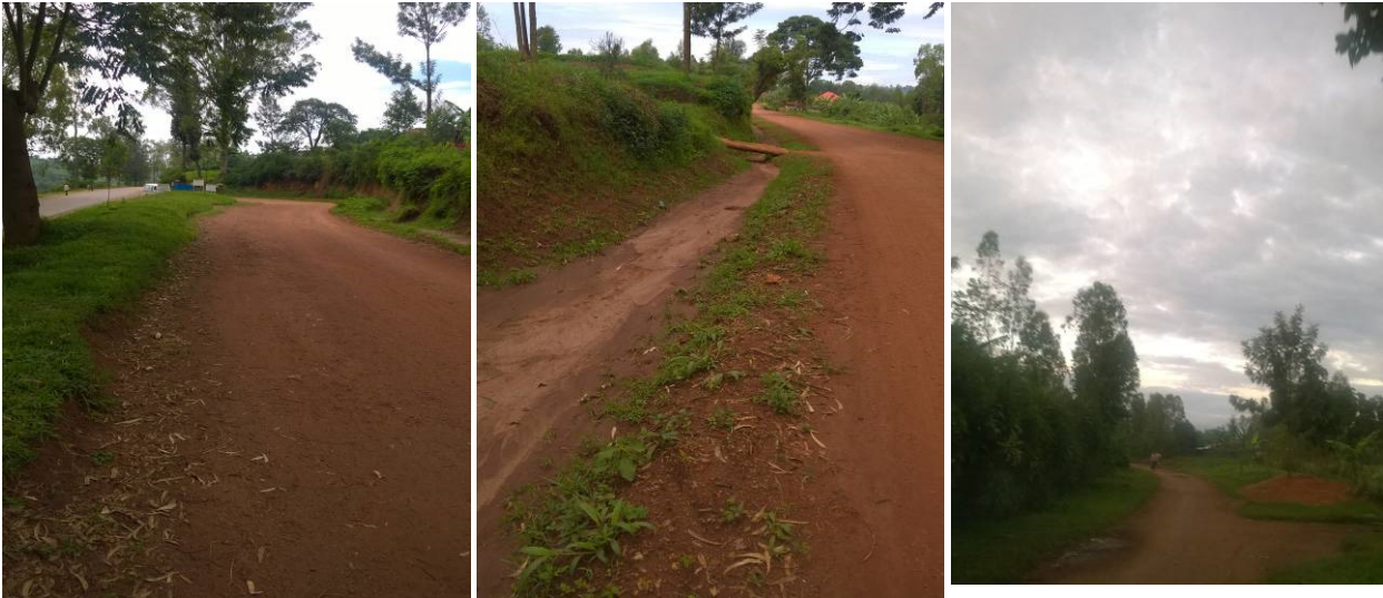
Plate 12: R31 proposed for rehabilitation to Mbazi Sector Office at Gatobotobo Cell and linking to National Road along Huye – Kigali Highway
