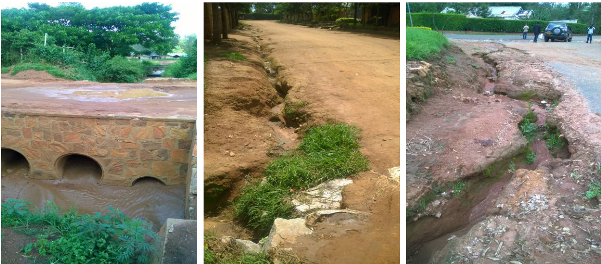
Plate 4: Drainage systems D1, D4, D5 and D6 need to be rehabilitated as their current state has resulted into storm water eating into the roads R2 and R1.
