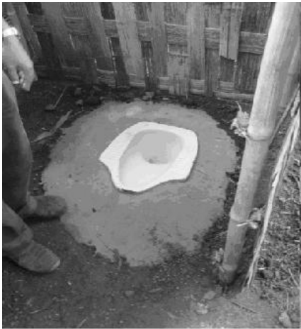
Four-flush latrine with air trap and ceramic pan without reservoir, Probolinggo district, August 2007.
