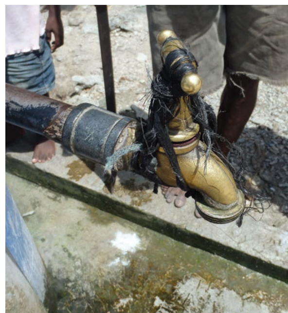
Figure 7. Inadequate Maintenance, Kamasina
