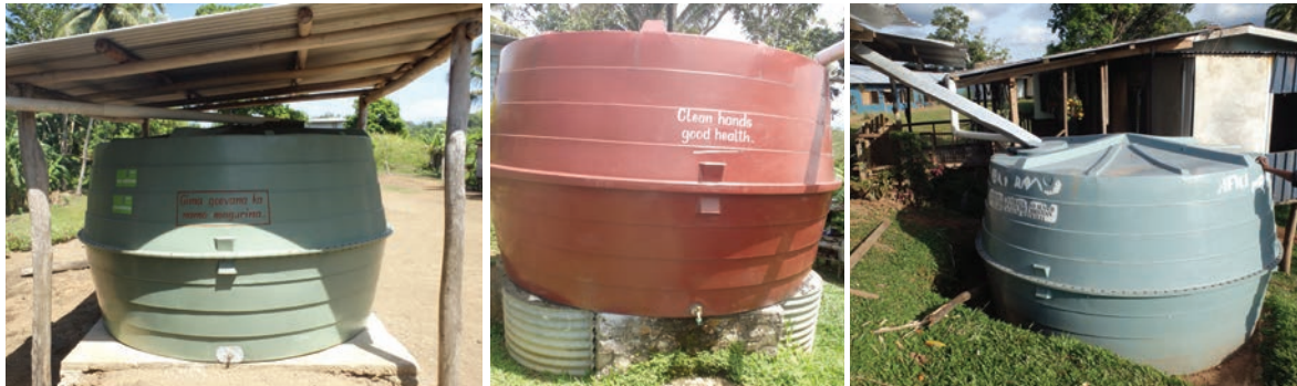
Figure 8. Rainwater Harvesting Systems, Gevera, Seba and Kokorogoro (Left to Right)
