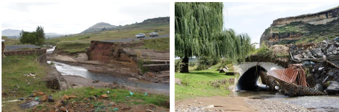
Figure: (left) Multiplate culvert washed away at Kubetu along B24 Road; (right) Flood damaged multi-plate culvert at Khukhune along A1 Road
