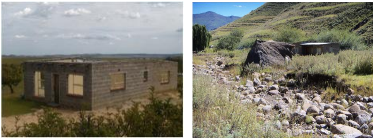
Figure: (left) De-roofed bungalow type of house in Kolonyama (Leribe district); (right) Houses located in or close to river beds (Botha Bothe district)
