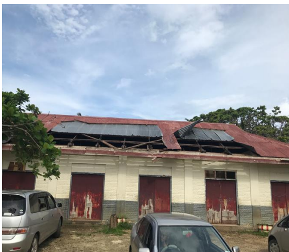
Figure 8 TC Gita: Major Roof Damage to Nuku'alofa Government Primary School
