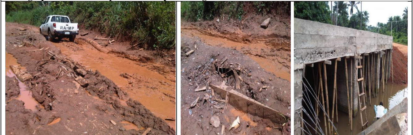
Failed portion of the road, construction of bridge, culvert.
