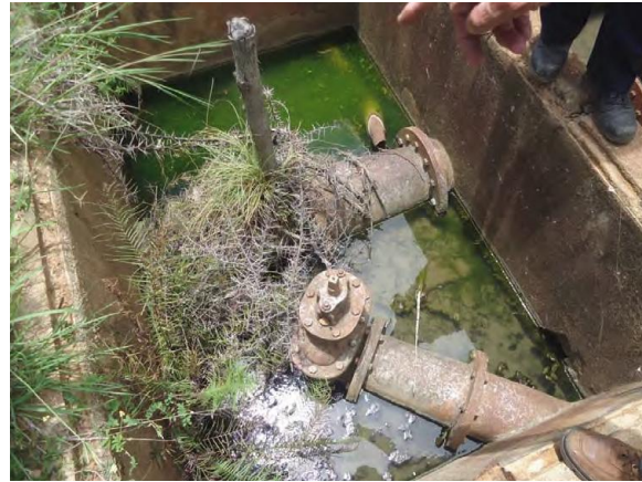
Ngondoma: Outlet pipe with a tree stump blocking a leak
