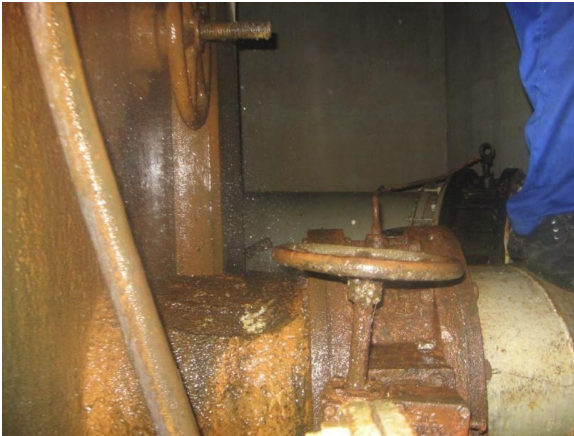
Mwenje: Rusted butterfly valve pipe
