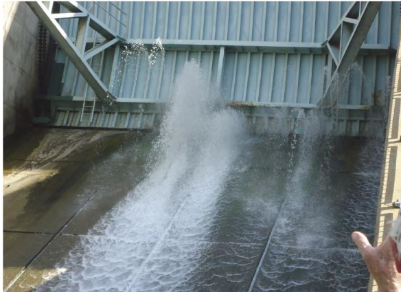
Manyame: Leakage in the radial spillway gate
