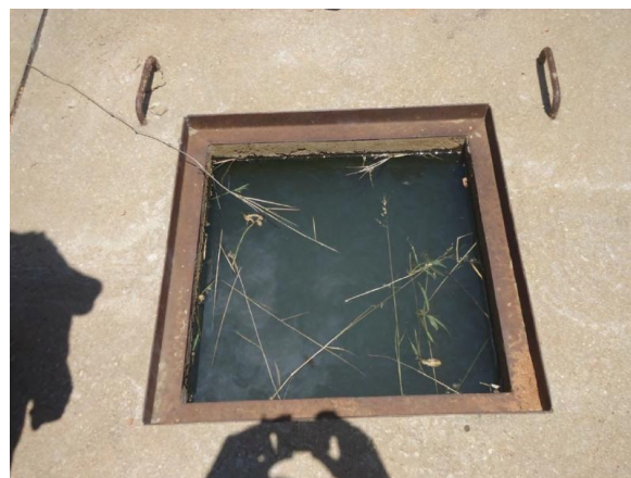
Mupudzi: Flooded valve house
