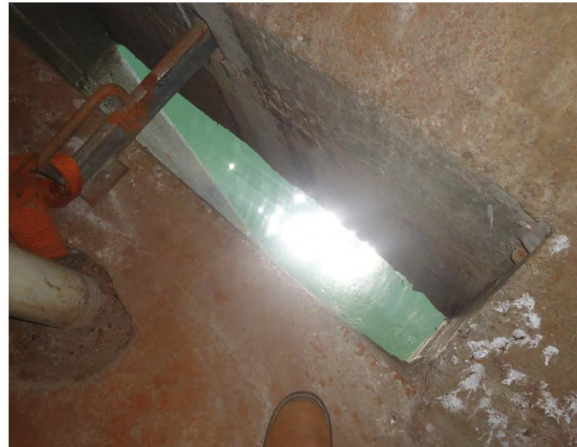
Osborne: Service gate stuck in half-open position
