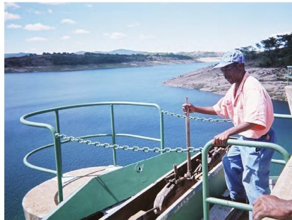
Mutirikwi: Manually operated dam gate mechanism
