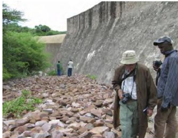
Lungwalala: Leakage from the left bank
