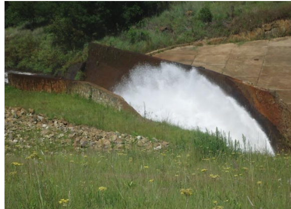
Smallbridge: Water gush from a jammed valve in the outlet
