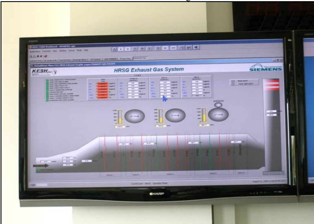
Photo 5. Readout of air monitoring station in operator room (indicative since plant not yet operational)
