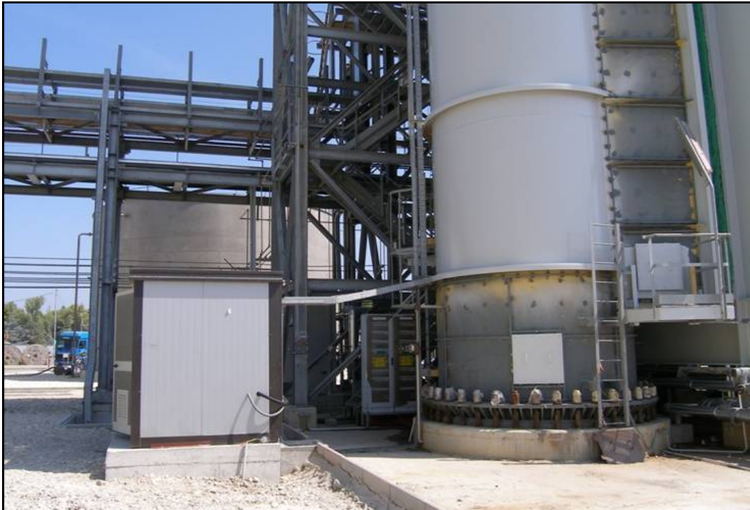
Photo 4. Continuous air monitoring station near stack
