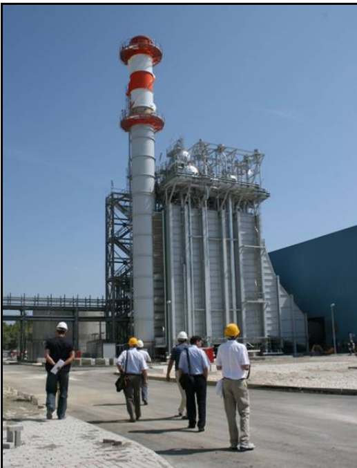
Photo 2. TPP inside facility area
