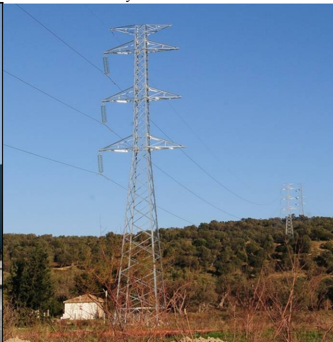
Photo 3. New transmission line
