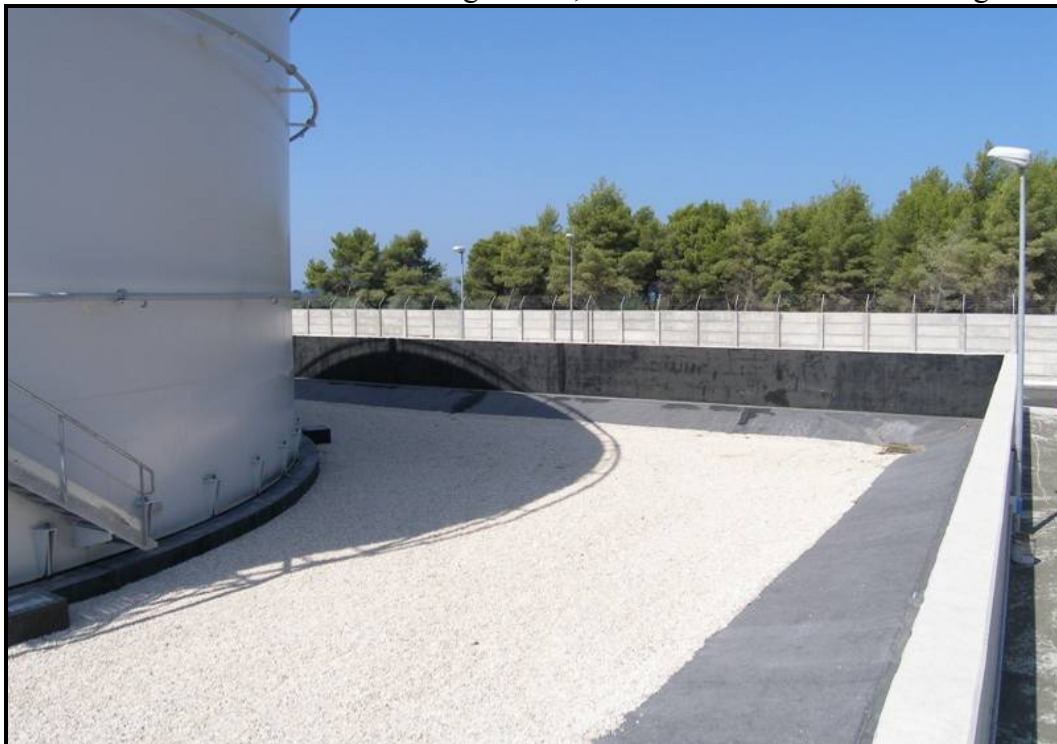
Photo 7. Spill containment around oil storage tank
