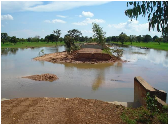
Rural Road Damaged by Ketsana
