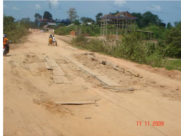
PR 2620 Damage after Ketsana
