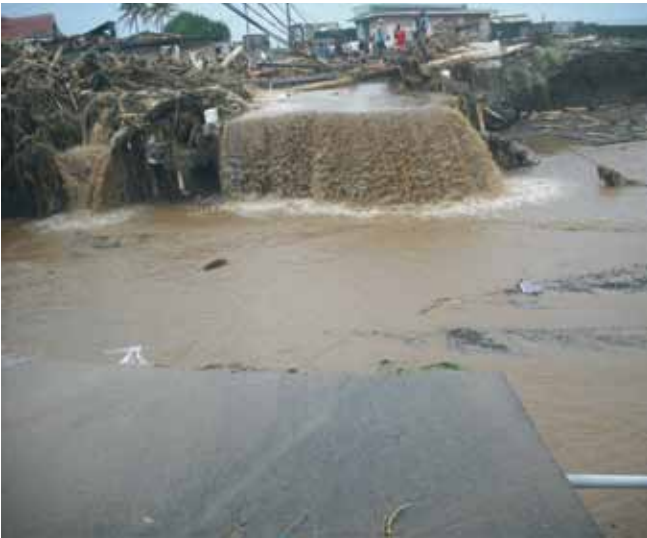
Road damage in Saint Vincent and the Grenadines after Hurricane Thomas in October 2010.
