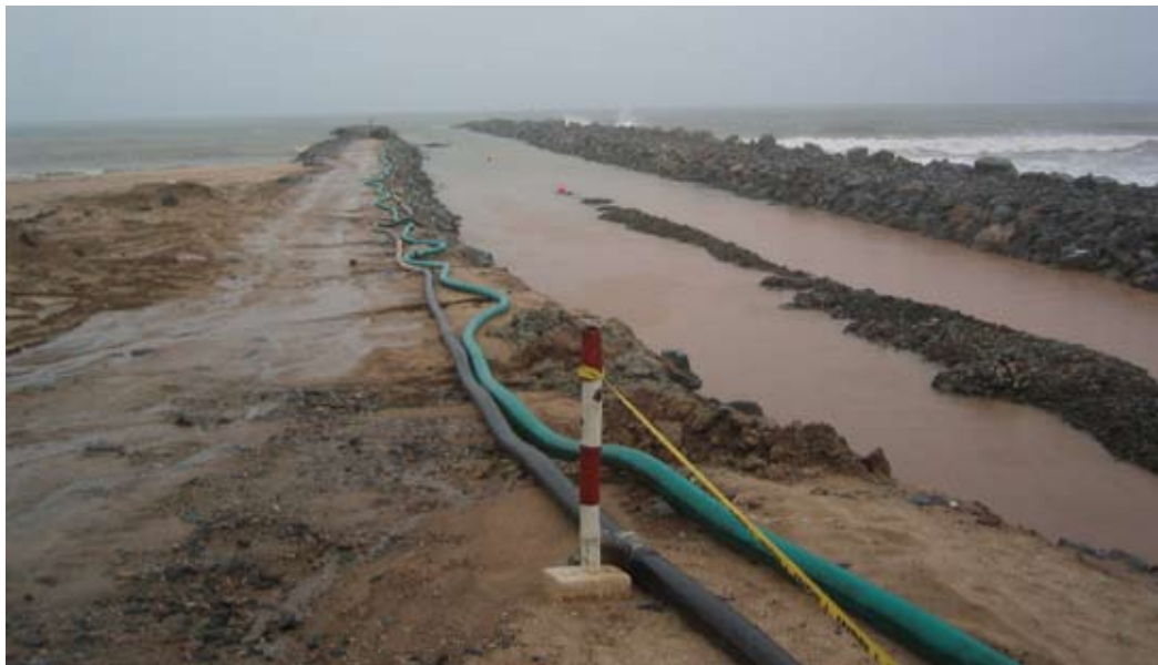
Nigeria: West Africa Gas Pipeline—Embankment protecting the gas pipeline as it reaches the shore of Takoradi in Ghana
