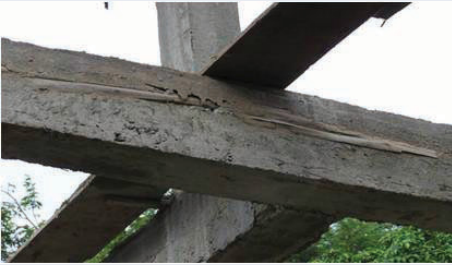
Figure 3.4 Debris embedded in a concrete support beam
