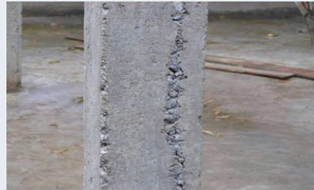
Figure 3.5 “Honeycombing” showing shoddy construction
