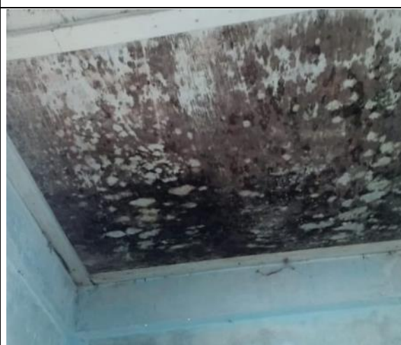
HCF quarter ceiling leakage, this is common in most HCFs
