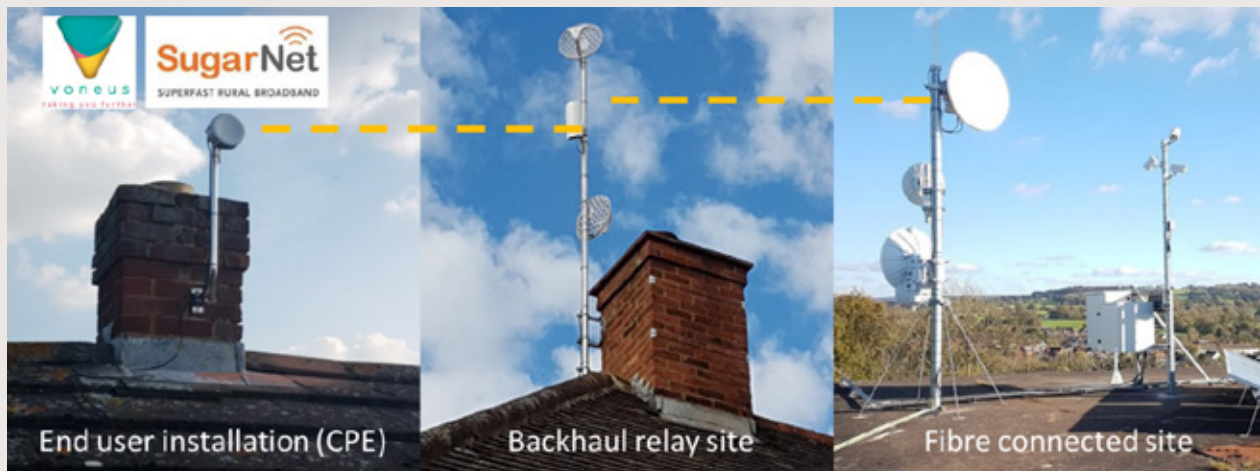
Figure B5.4.1: SugarNet/Voneus Mixed Fiber-Wireless Solutions for Delivering Rural Broadband Connectivity in the United Kingdom
