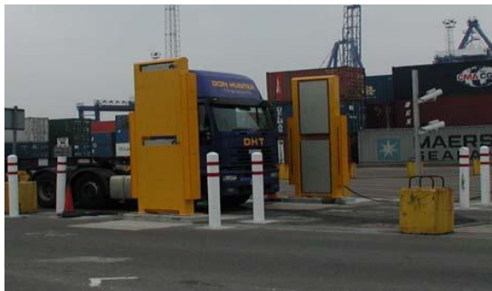
Radiation Portal Monitors installed at Port of Felixstowe (UK).
