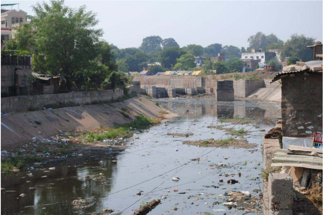
Photo 4. October 2010: Accumulation of debris due to lack of cleaning
