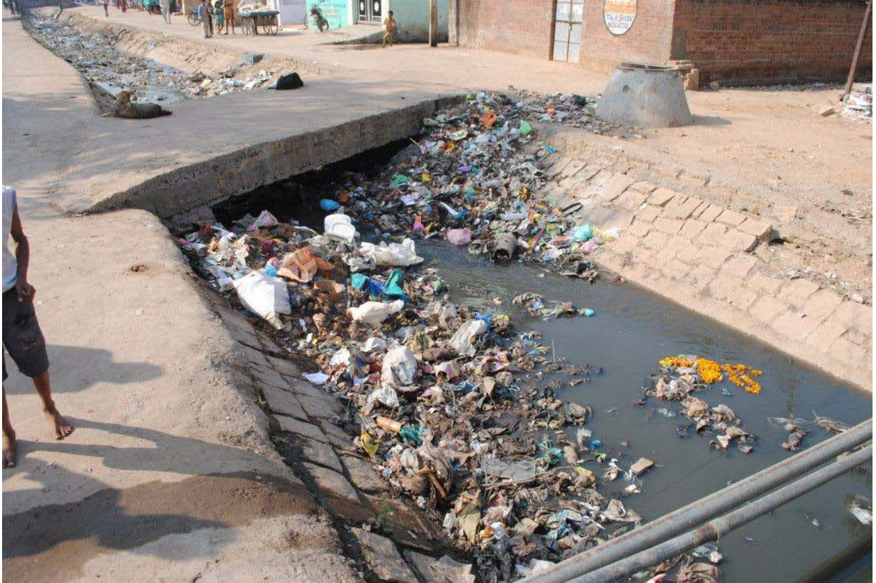
Photo 3. October 2010: Accumulation of debris in a Nalla due to lack of cleaning
